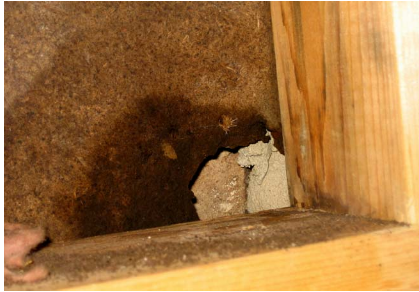
Photo - Hole in sheathing below dining room window.
