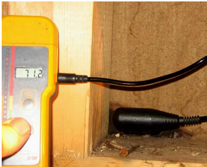
Photo - Moisture reading below dining room window
