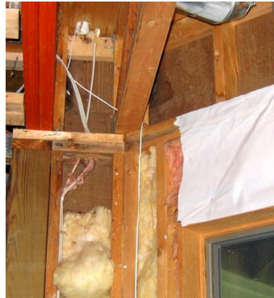
Photo - Rear wall water entry locations
