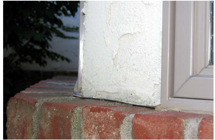
Photo - Dining room corner, caulk and flashing
